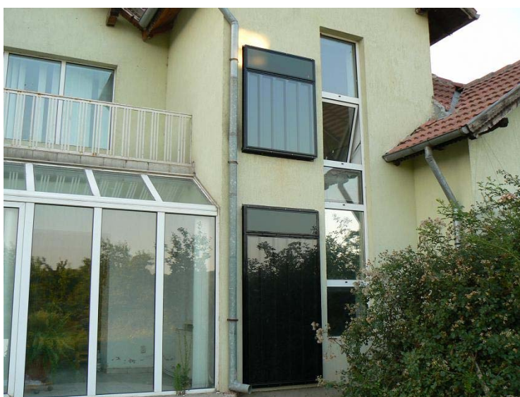
Montare verticala panou solar 1000G si panou solar 1500G in Branesti – Bucuresti
